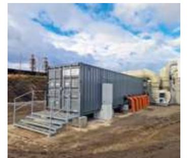
Control container for monitoring the composting process.
