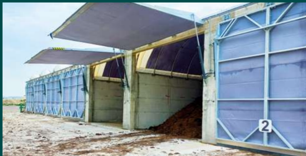
The material enters a box closed by a hinged door for the first phase of composting, namely sanitization.
