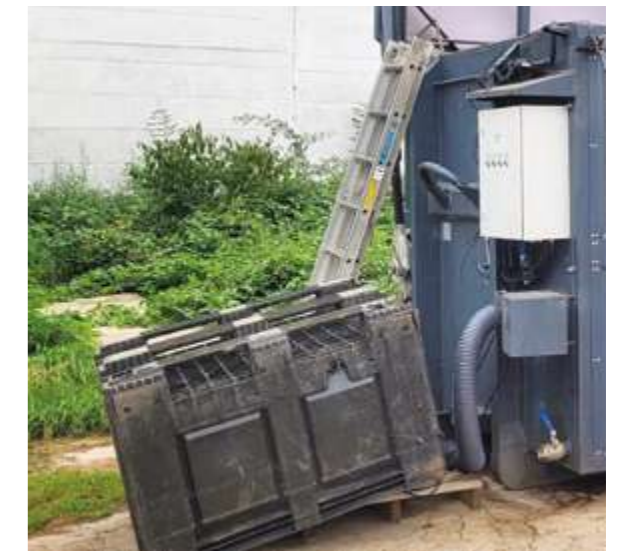
230 V aeration fan connected via quick coupling.
