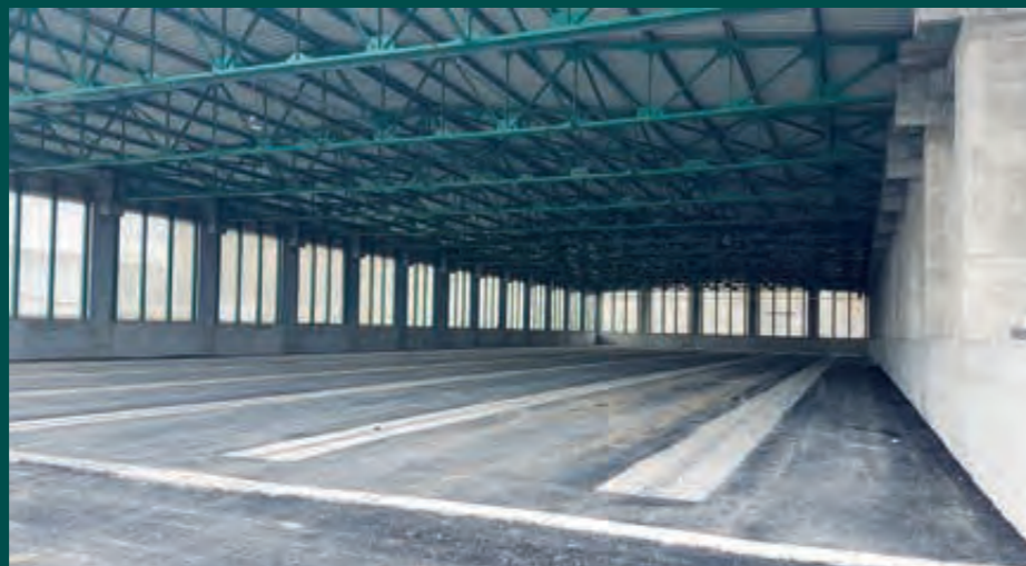
A completed compost facility at the Tripoli plant.
