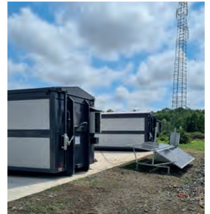
CSC-Containers and PV system
